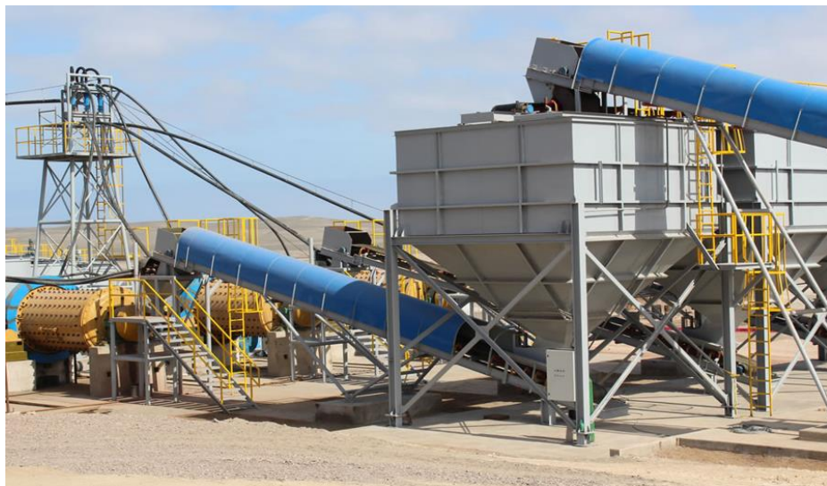
Kori One plant - Ball mills and Crusher circuit
