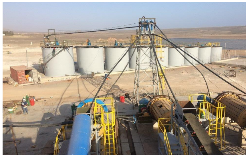
Kori One plant - Tanks
