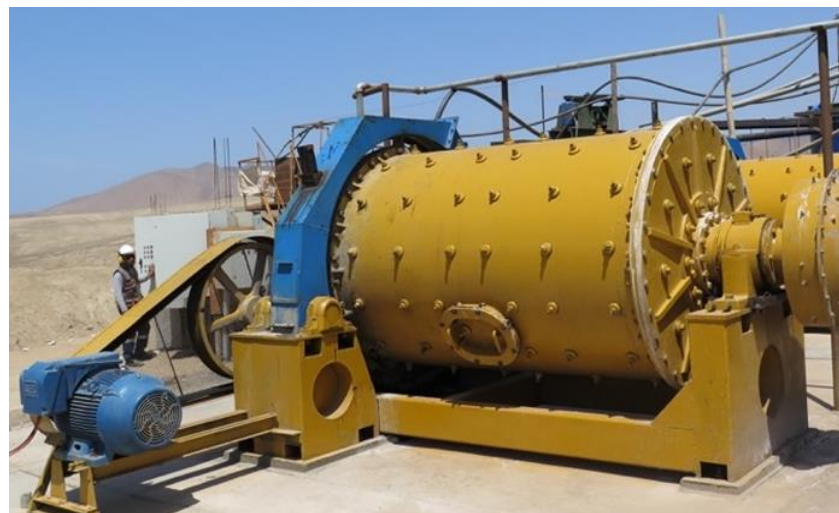
Chala One plant - Ball mills
